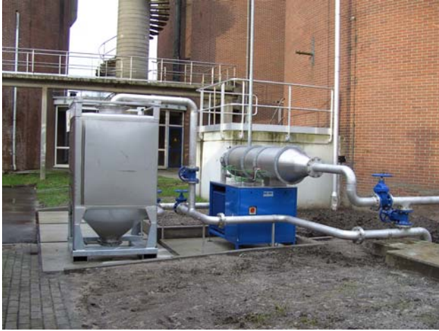
PROJECT RWZI ASSEN ➤ CONDITIONERING BIOGAS
